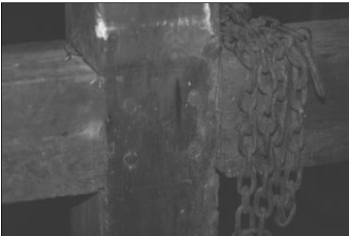
The old historic barns built in the late 1800s and into the 1900s had elaborate systems of wooden posts, beams, and braces, all fastened together with wooden pegs, shown here and above.
